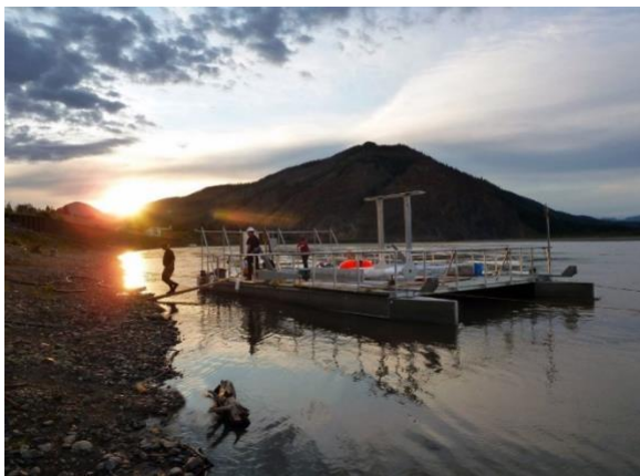
Fig. 4 Preparing for installation of a 25kW low flow unit on the Yukon River, Alaska
